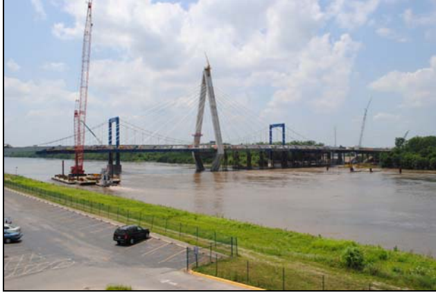
Only eight stay-cables are left to install before the bridge is complete.
