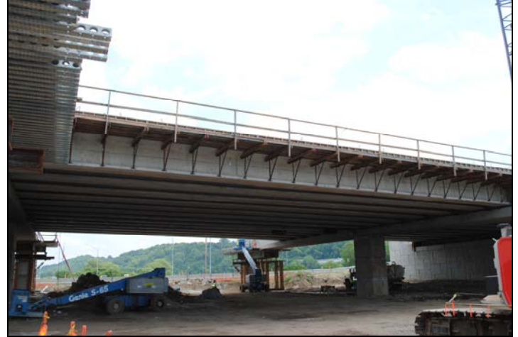
Work continues on the single-point urban interchange at I-29/35 and Front Street. Traffic is scheduled to be back on the mainline interstate (and off the temporary ramps) by Fall 2010.
