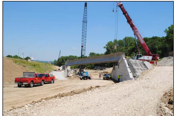
Missouri's three longest concrete bridge girders were recently set in place for the Paseo Boulevard off-ramp, near Independence Avenue. Each girder weighs approximately 150,000 pounds and is around 150 feet long.
