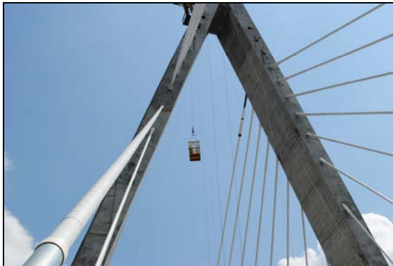
River Bridge progress continues. With 32 stay-cables installed and paving work largely complete on the north and south approaches to the pylon; work is moving as swiftly as the Missouri River currents. (Photo provided by David Woods with Paseo Corridor Constructors.)
